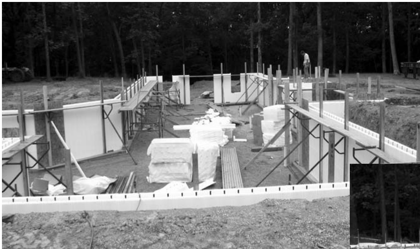
Left: Brad Doll used Integraspec Insulating Concrete Forms for the upper and lower levels of his 3000 sq. ft. concrete home.
