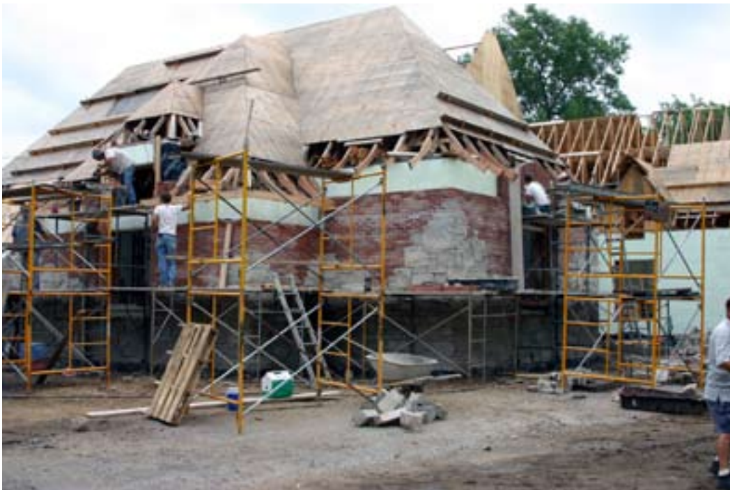
400 yards of above grade concrete goes into this ICF home outside Lincoln, IL.
