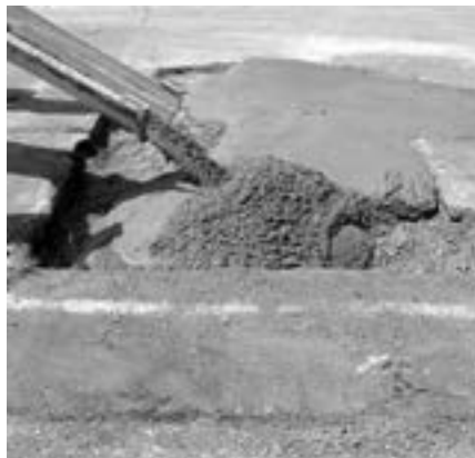
Flowable fill is used to fill voids in the current pavement of the Long John Silver parking lot in Peoria, IL.
