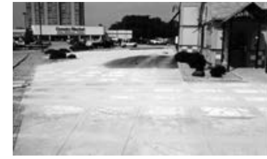
Far left: The Long John Silver parking lot prior to Ultra-Thin Whitetopping overlay.
