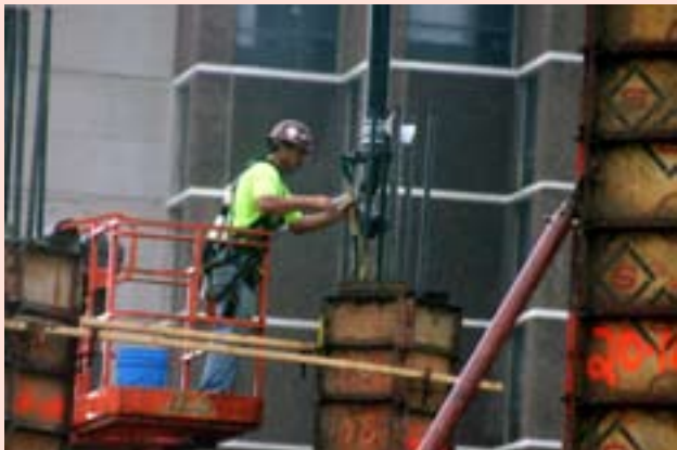
A laborer in a lift bucket directs SCC into tall forms on a jobsite in downtown Normal.
