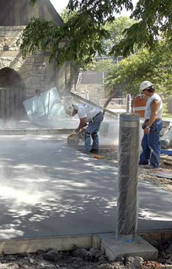
Clockwise from left: A gray powder is put on the colored concrete before it is stamped (photo courtesy of The Pantagraph ); A view of Ewing Manor during the construction of the Genevieve Green Gardens at the Ewing Cultural Center in Bloomington; The red running cobblestone courtyard on the east side of Ewing Manor.
