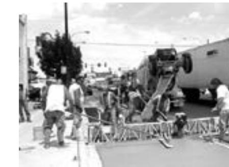
Bus pads on Western Avenue are paved using vibrating screeds and a special concrete mixture containing 7.5 lbs. per cubic yard of synthetic structural fibers.
