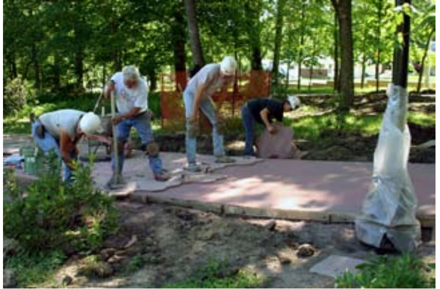
Pictured below are workers stamping the cobblestone path and the cobblestone path upon completion.
