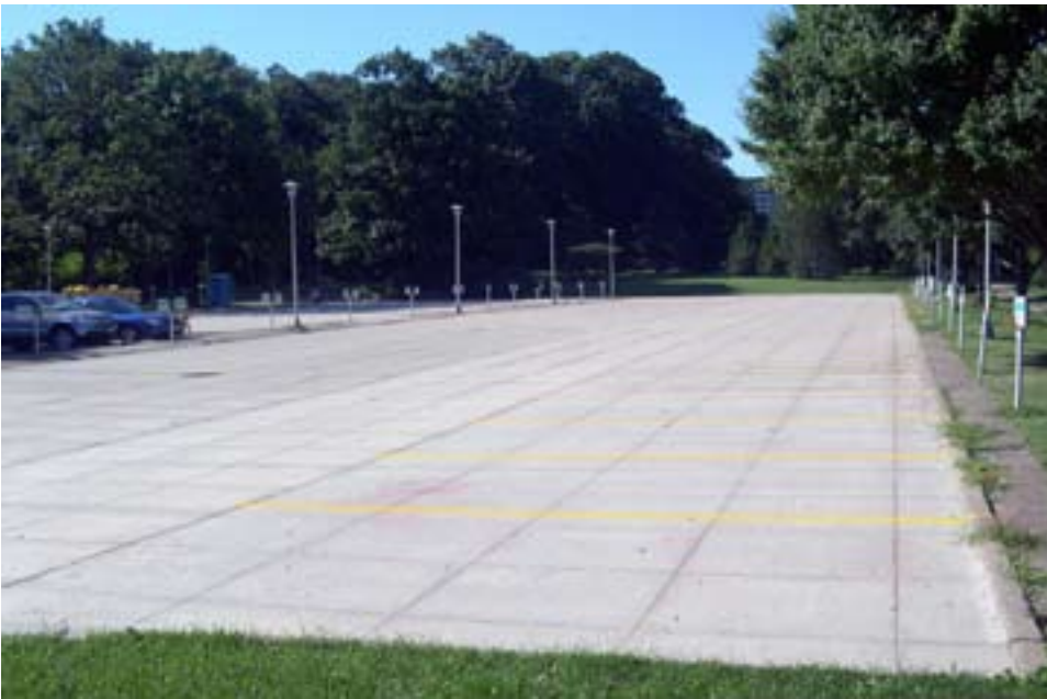
A parking lot overlay at the University of Illinois Urbana-Champaign. Notice the jointing pattern.
