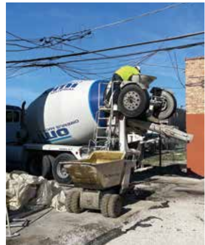
A load of concrete gets color admixture at the South Side Sanctuary project.
