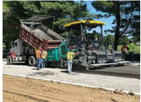
CCP mix is delivered in standard dump trucks, dumped into the hopper, and placed in the same fashion as standard HMA mixes.
