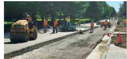
After placement through the high-density paver, CCP is rolled, tested for compaction, finished, and cured, all in concurrent order.
