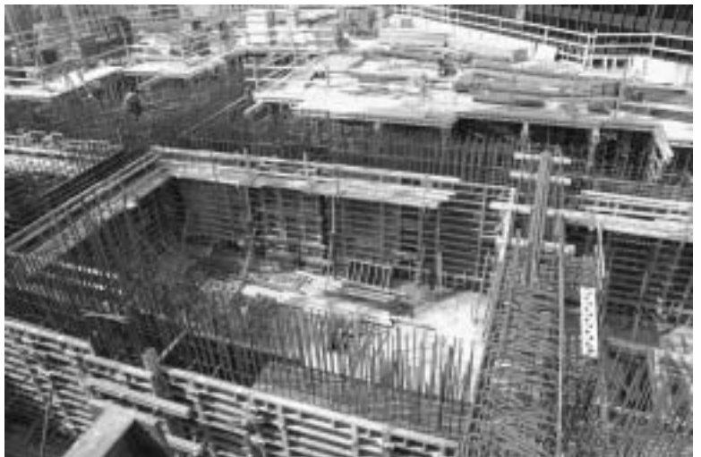
A view of the steel used in the all reinforced concrete structure.
