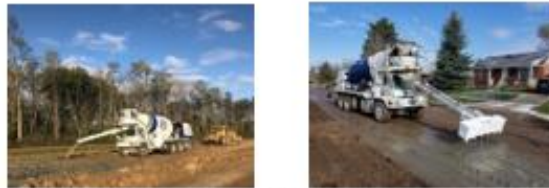
Figure 1. Spreading cement slurry from a ready mixed concrete truck (Photos courtesy Scott Hall, Sagamore Ready Mix, left; Dr. Spencer Guthrie, BYU, right)
