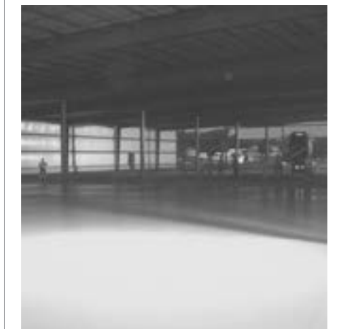
The first pour of the project nears completion. Using a laser screed affords an extremely smooth surface.
