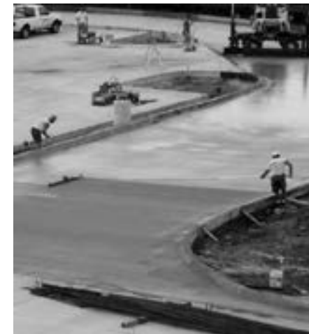
Pictured above: Texturing the wide placement required an additional worker to move the broom.
