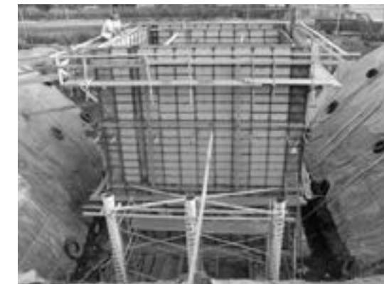
Left: Workers complete inspection on the 24' wall prior to the Self Consolidating Concrete pour. The wall is loaded with rebar and several boxouts at different elevations.
