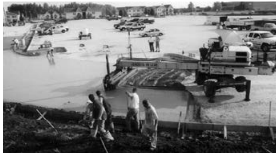
Pictured above: The Kerasotes project included curb to curb concrete placement. The pile of concrete in the foreground was used to build the integral curb.
